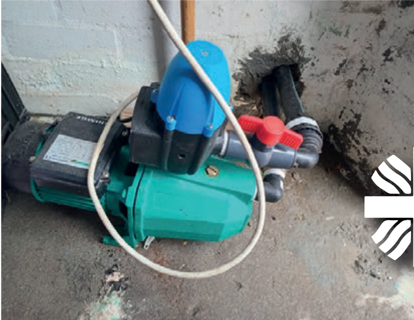
Figure 11 – Water pump sponsored through CCT Kommetjie parish grant
